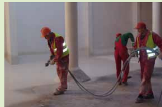
Drinking water tank, Tarnów, Poland
