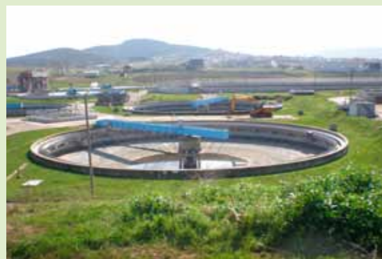
Sewage treatment plant, Istanbul, Turkey
